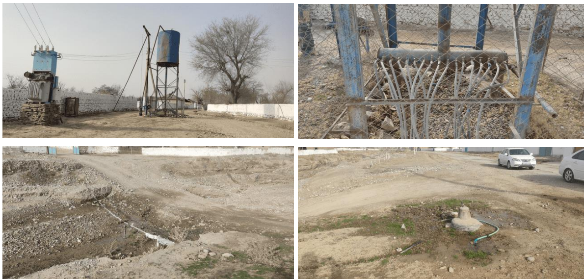
Figure 1. An existing water supply system in RCA Koshtal
